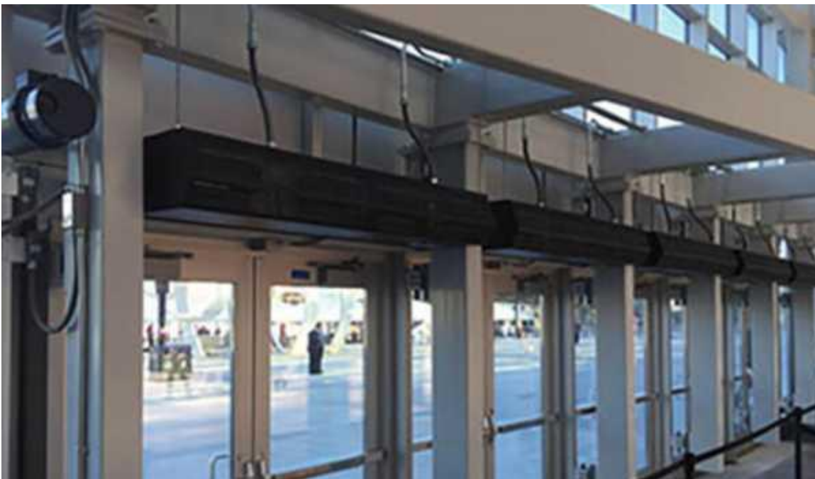
Foto A: Perdele de aer instalate la U.S. Bank Stadium Minneapolis. Credit: Mars Air Systems
